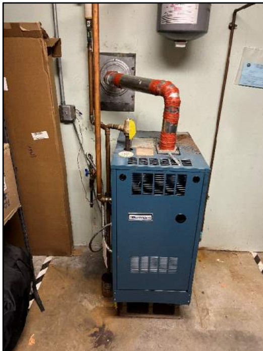
Boiler located in the cell and holding area.
