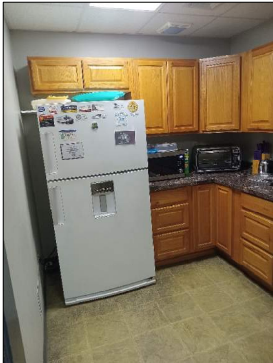
Heavily Worn Flooring Tile in Kitchenette.
