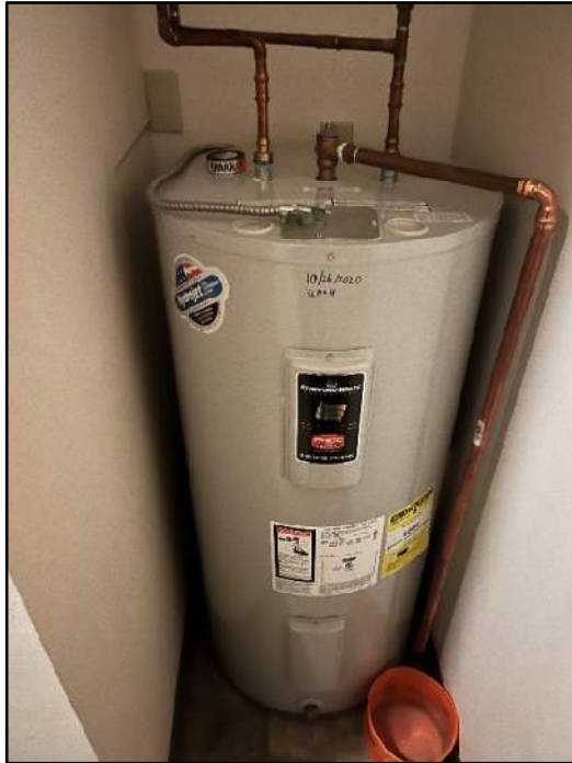
Hot water heater serving the locker room/bathroom spaces.
