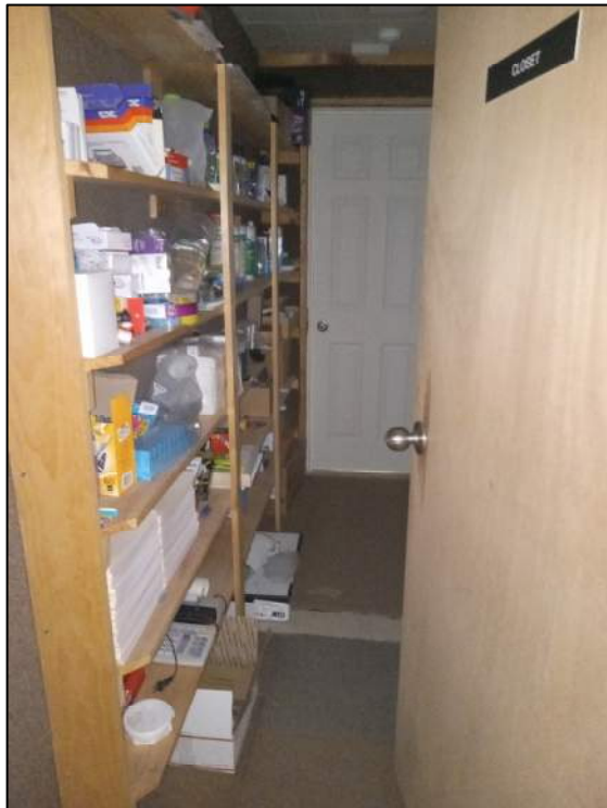
Not Permanent Floor Finish on Concrete Floor Slab in Closet.
