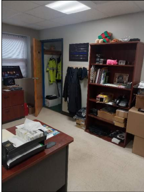
Worn and Stained Flooring Tile in Offices.
