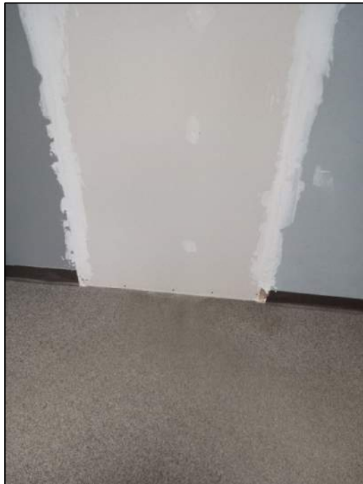
Unfinished Infilled Opening in Women's Restroom.
