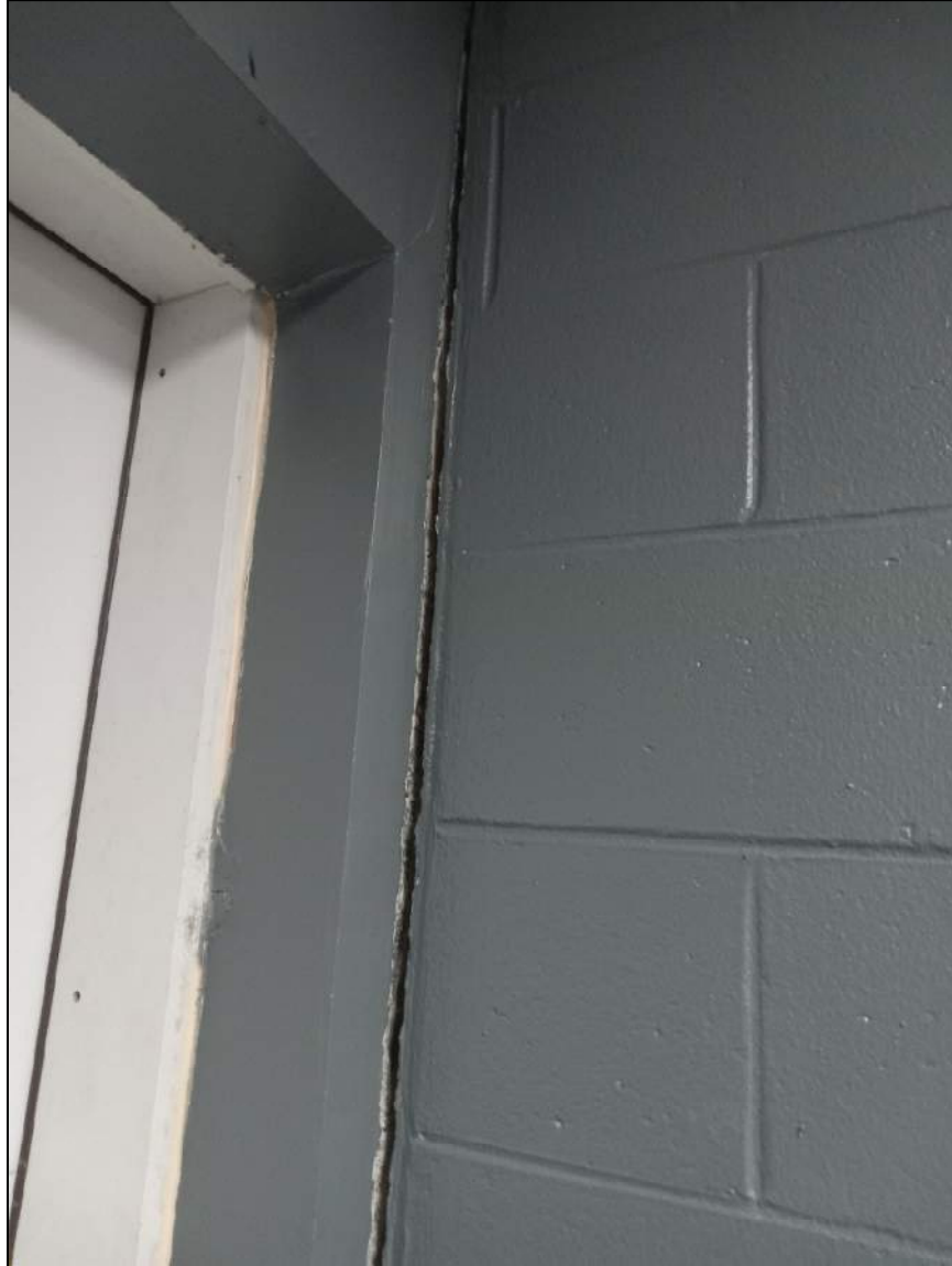
Concrete Masonry Wall Separating from Adjacent Concrete Wall at Armory.
