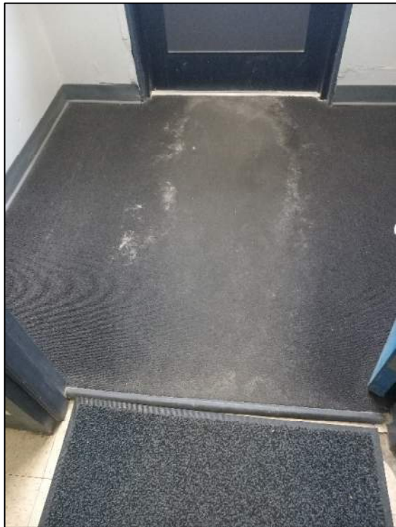
Heavily Worn Carpet Floor Finish in Exit Vestibule.
