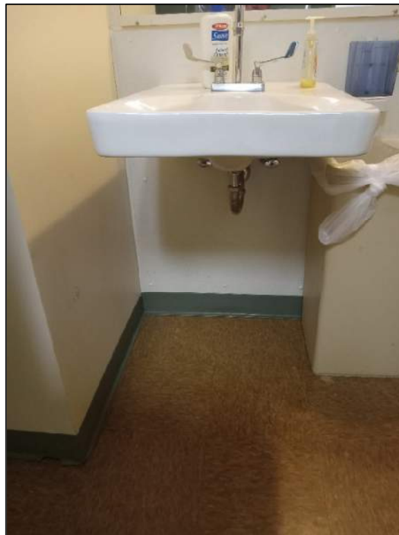
Missing Insulation at Accessible Sink Waste Pipe in Women's Restroom.
