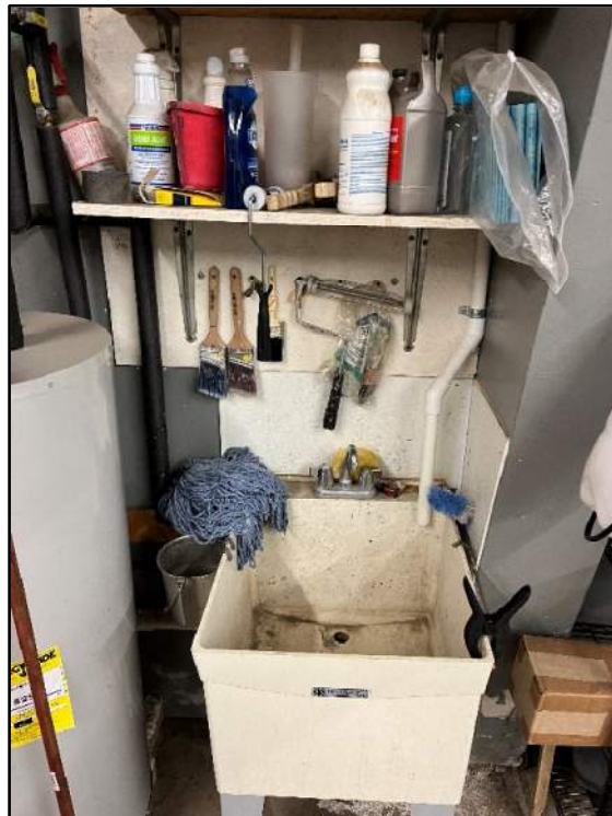
Service sink located in the garage area.
