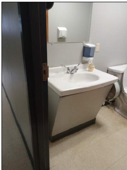
Mirror is Mounted too High Above the Floor.
