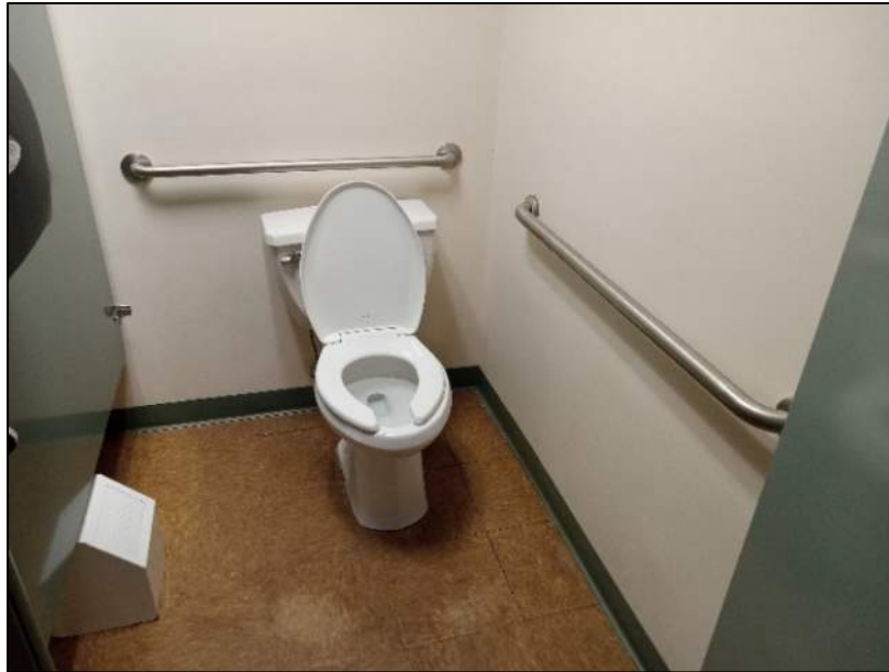
Missing Vertical Grab Bar at Side Wall of Accessible Toilet Stall in Women's Restroom.
