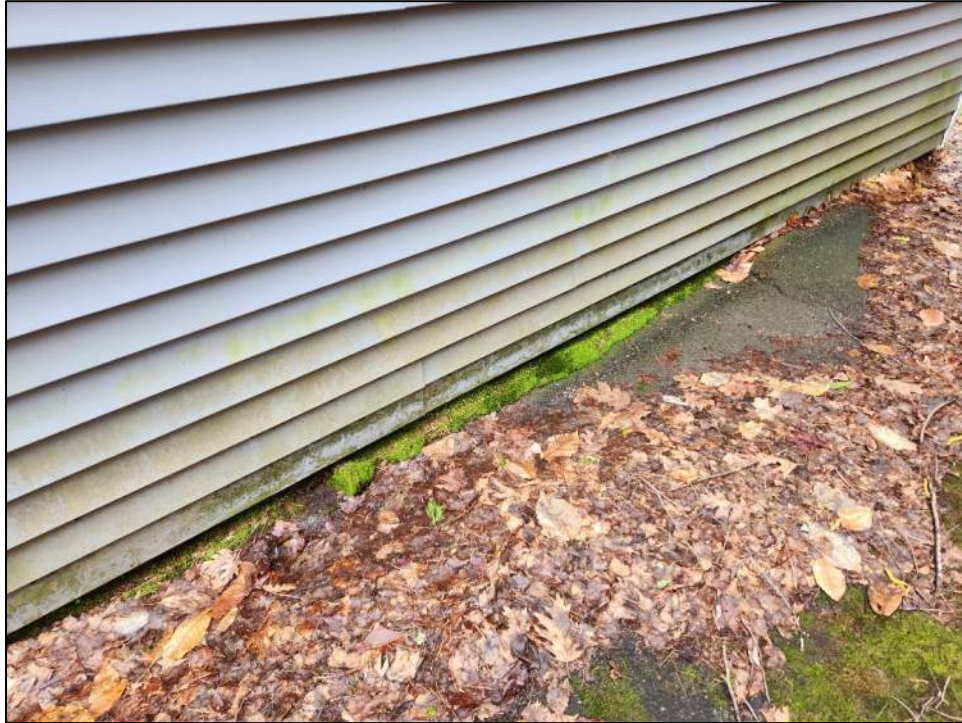
Moss Growing and Stained Siding along the Rear of the Building.
