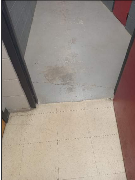
Missing Flooring Transition.
