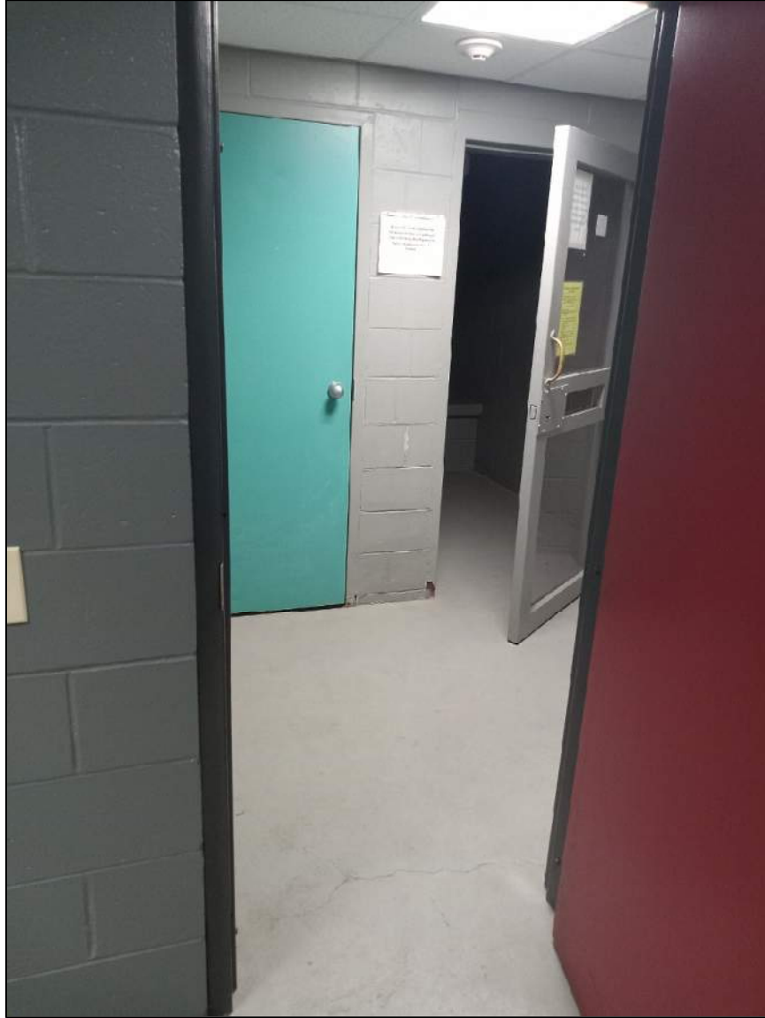
Damaged Metal Door Frame at Bottom of Juvenile Cell Door.
