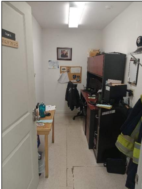
Patched Flooring Tiles.
