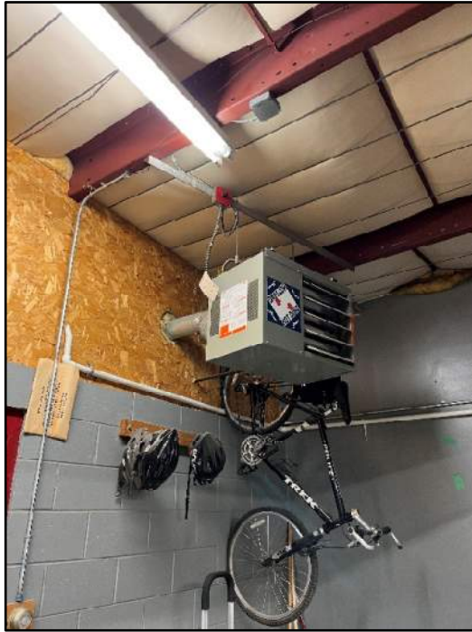
Modine Hot Dawg unit heater in the garage area.
