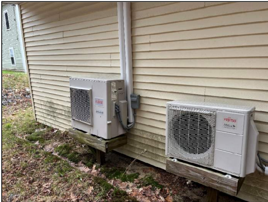
Additional condensing units for the office heat pump units on wooden risers.
