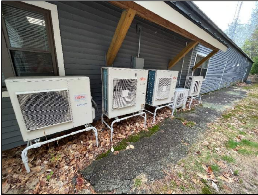
Condensing unit for all the interior heat pump units.
