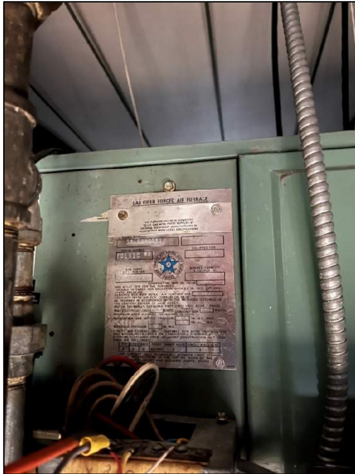
Existing gas-forced hot air furnace in the plenum space.
