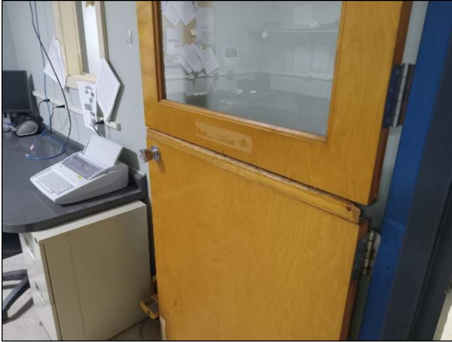
Damaged Dutch Door at State Police Office.
