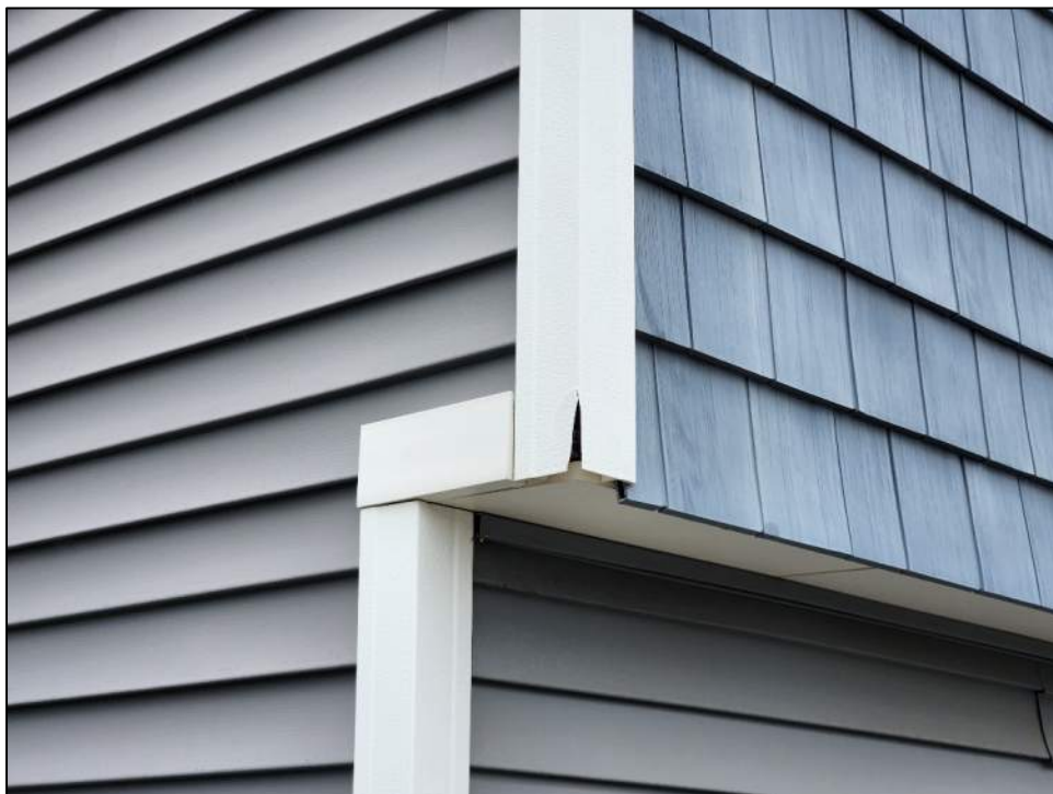
Cracked Corner Board.
