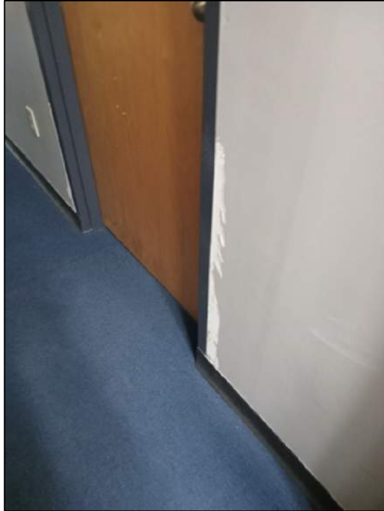
Damaged Wall Finish Surfaces Adjacent to Interview Room Door.
