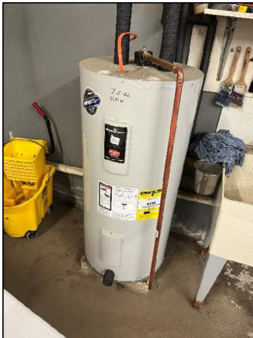
Hot water heater located in the garage area.
