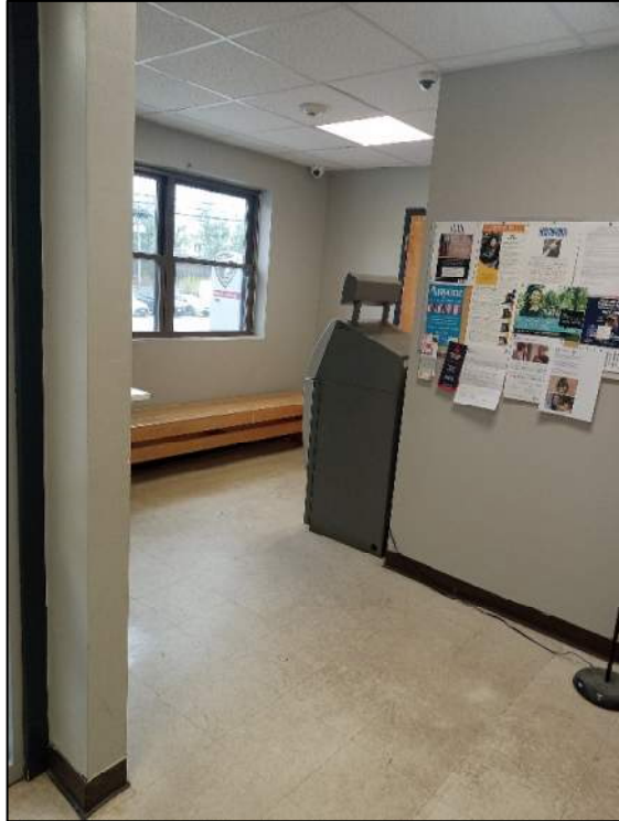
Heavily Worn Flooring Tiles in Public Waiting Area.
