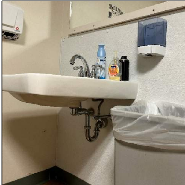
Bathroom sink requiring Lavguard for ADA compliance.
