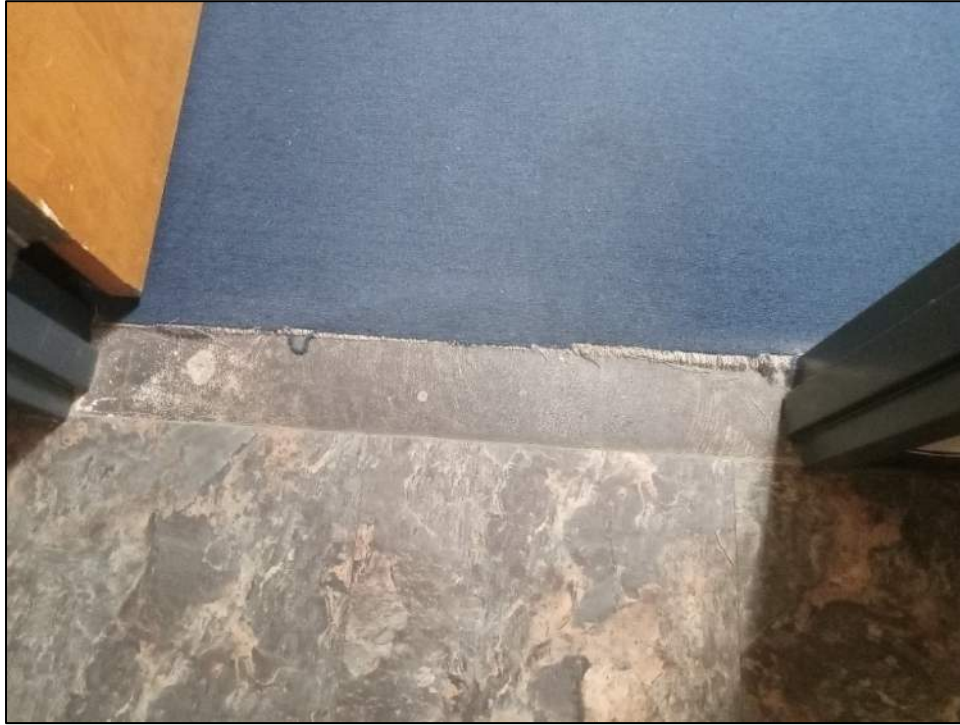
Exposed Concrete Floor Slab at Missing Flooring Transitions.
