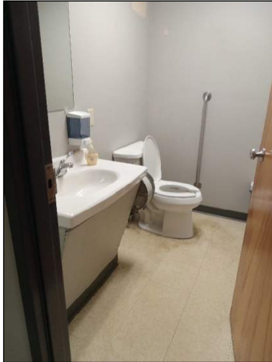
Missing Horizontal Grab Bars at Back Wall and Side Wall in Accessible Public Restroom. Insufficient Space Between Toilet and Sink for Wheelchair Maneuvering.
