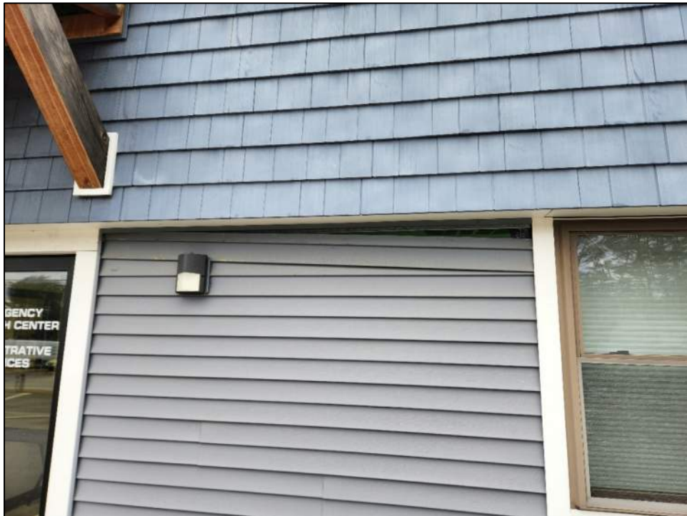
Damaged Siding Adjacent to Front Entry.
