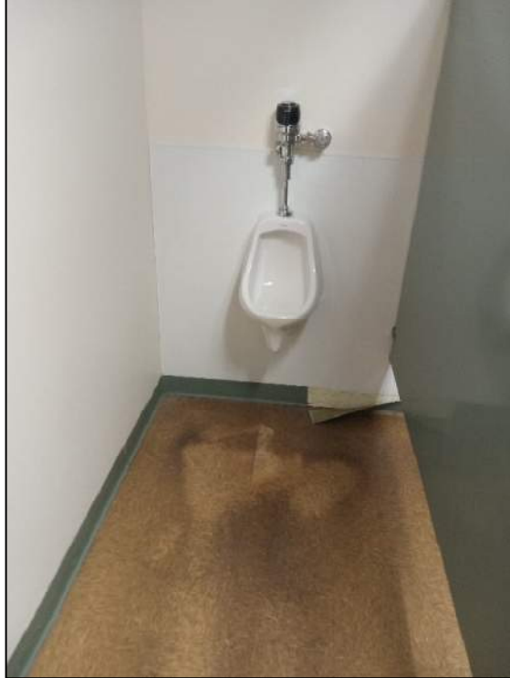
Heavily Worn Flooring Tile and Peeling Vinyl Baseboard in Men's Restroom.
