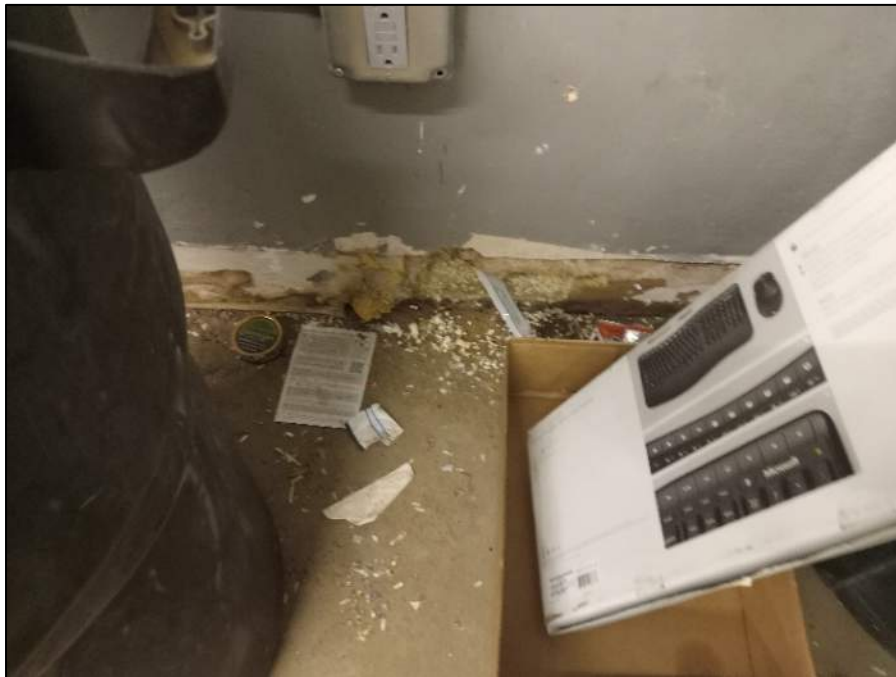
Damaged Gypsum Wallboard and Missing Baseboard at Bottom of Wall in Sallyport.
